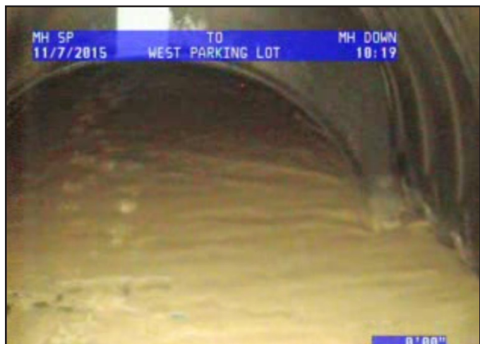
SEPARATOR ROW: Separator Row prior to cleaning
